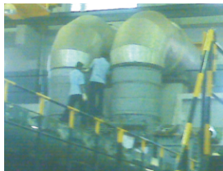
bellow covers at power plant
