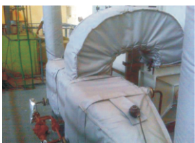
Removable Insulation for equipment
